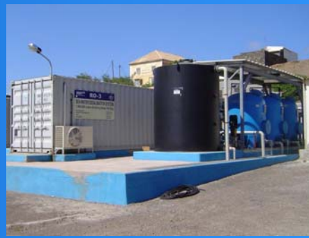
Reverse Osmosis Units
