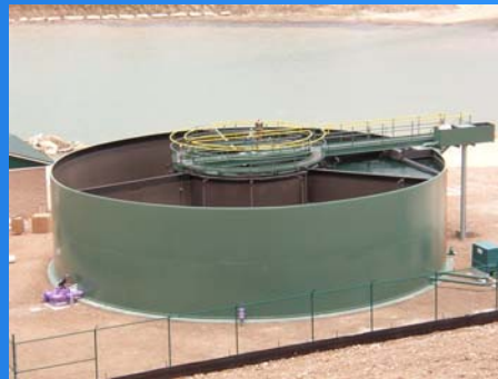
Field Erect Wastewater Treatment System
